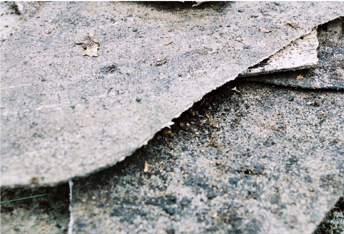
5/12/06 Photo Showing Asbestos Fibers on the Edges of Debris
