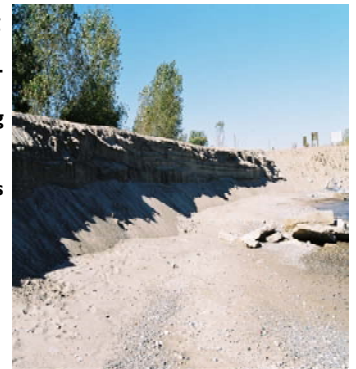
October, 2004 Erosion of contaminated sand pile (regulated waste) before the winter storms. How much more is now mixed into the sand or washed into the lake?
