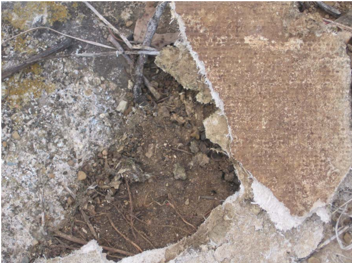
Figure 2 - Notice the toxic asbestos fibers protruding along the edges of the friable debris
